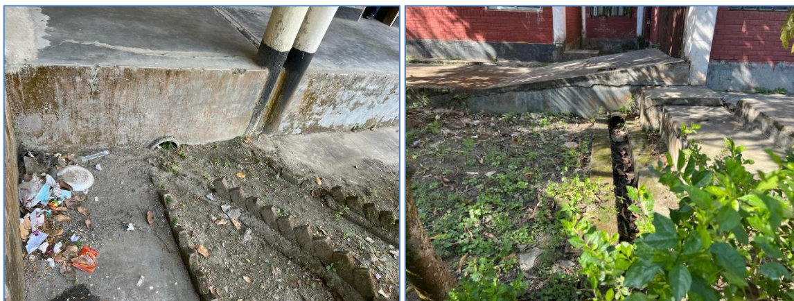
Figure VI-10 Images of the current drainage system at the proposed NATI site. Photo: TA consultants
