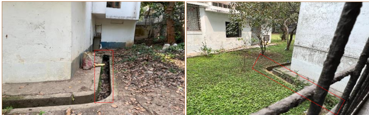
Figure III-4 Drainage system is either non-existing or non-functioning within the IBA campus.
