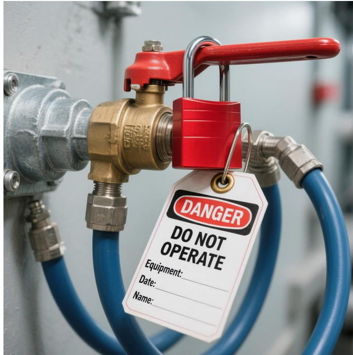
Figure 8.1: Example of a Lock-Out/Tag-Out on a pneumatic shut-off valve.
