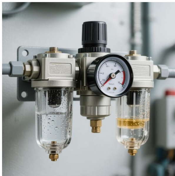
Figure 8.2: Inspecting the FRL unit. The filter bowl on the left clearly shows accumulated water that needs to be drained.
