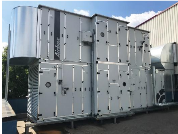
Fig: Air Treatment Plant
